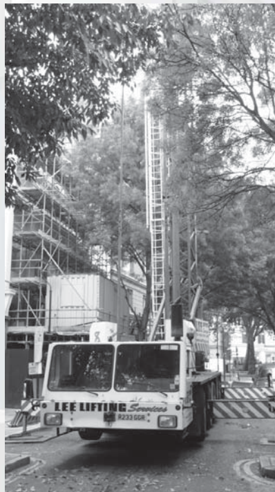
Crane for lifting up the air handling unit to the back of the church
