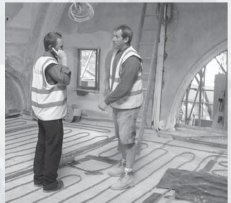
Nick Smith, Site Manager (Saltash), Paul Corrigan, Laid underfloor heating pipes on the gallery floor
