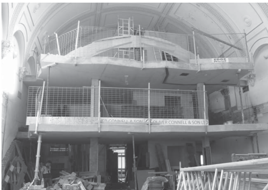
All concrete floors built and fully visible at the end of July 2009
