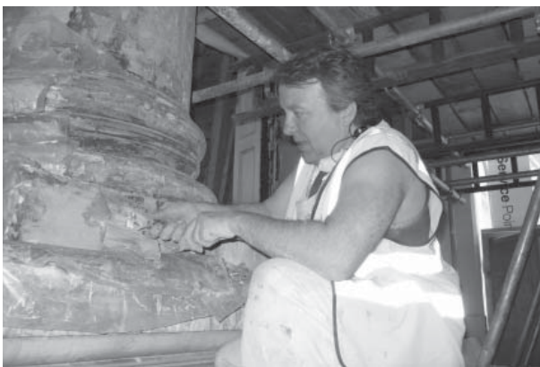
Andy Bradley (Saltash) removes multiple layers of paint on the external facade with his spatula
