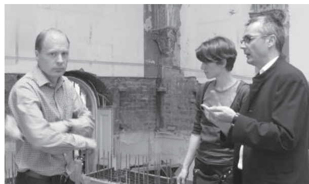
Site meeting: Architects Mark Cleveland (WCP) and Stephanie Hirschvogel (Christ & Gantenbein) and Project Manager Rolf Peruzzo (Castle Davis)
