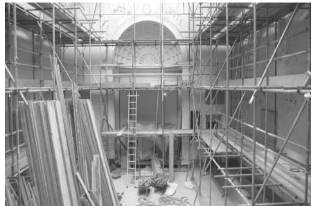
Interior scaffolding erected to replace roof lights and to do interior decoration
