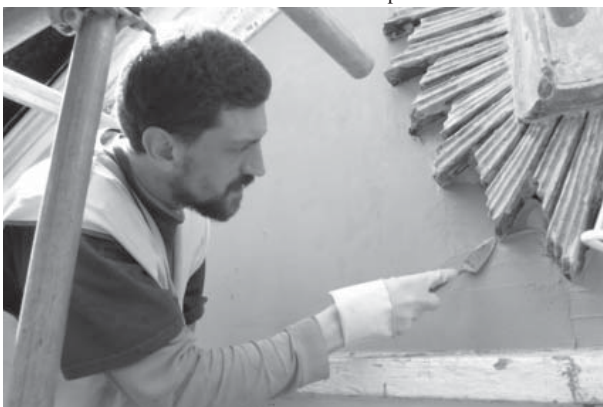
Matthew Finnagen (Finnagens Stone Work Restoration) smooths a second coat of rendering
