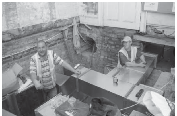
Jason Chevis and Simon Cox (Wandle Plumbing) putting in stainless steel ventilation ducts
